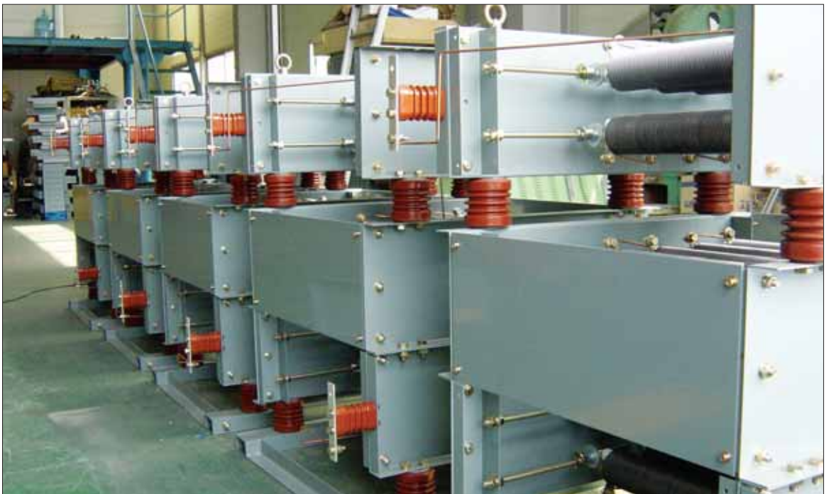
NGR(Neutral Grounding Resistor)
